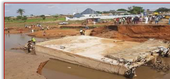
Figure 3. Alagbado bridge along Foma–river washed away by the flood.
