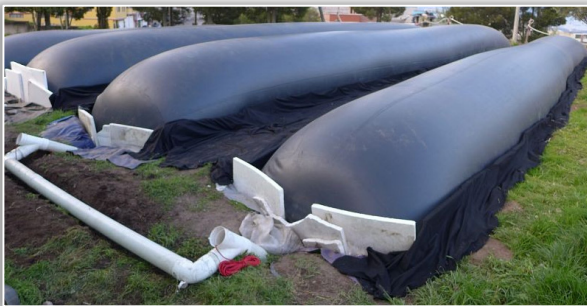
Figure 10 – Tubular biodigesters for slaughterhouse wastewater ( www.wisions.net )
