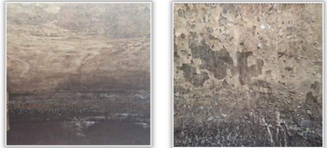
Figure 8. Chemical attack on the inner surface
