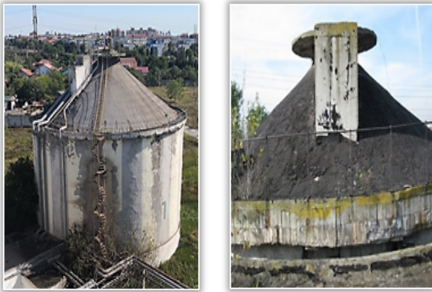
Figure 6. Cylindrical-conical fermentation tanks with cracked roof dome
