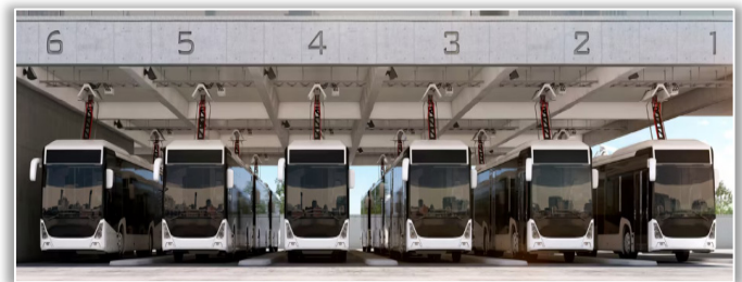
Figure 5. ABB pantograph e-bus charging system
